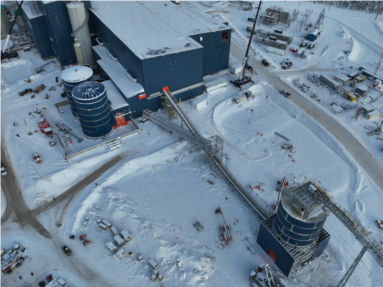
Crushed Ore Conveyor and Process Plant (Middle of December 2025)
