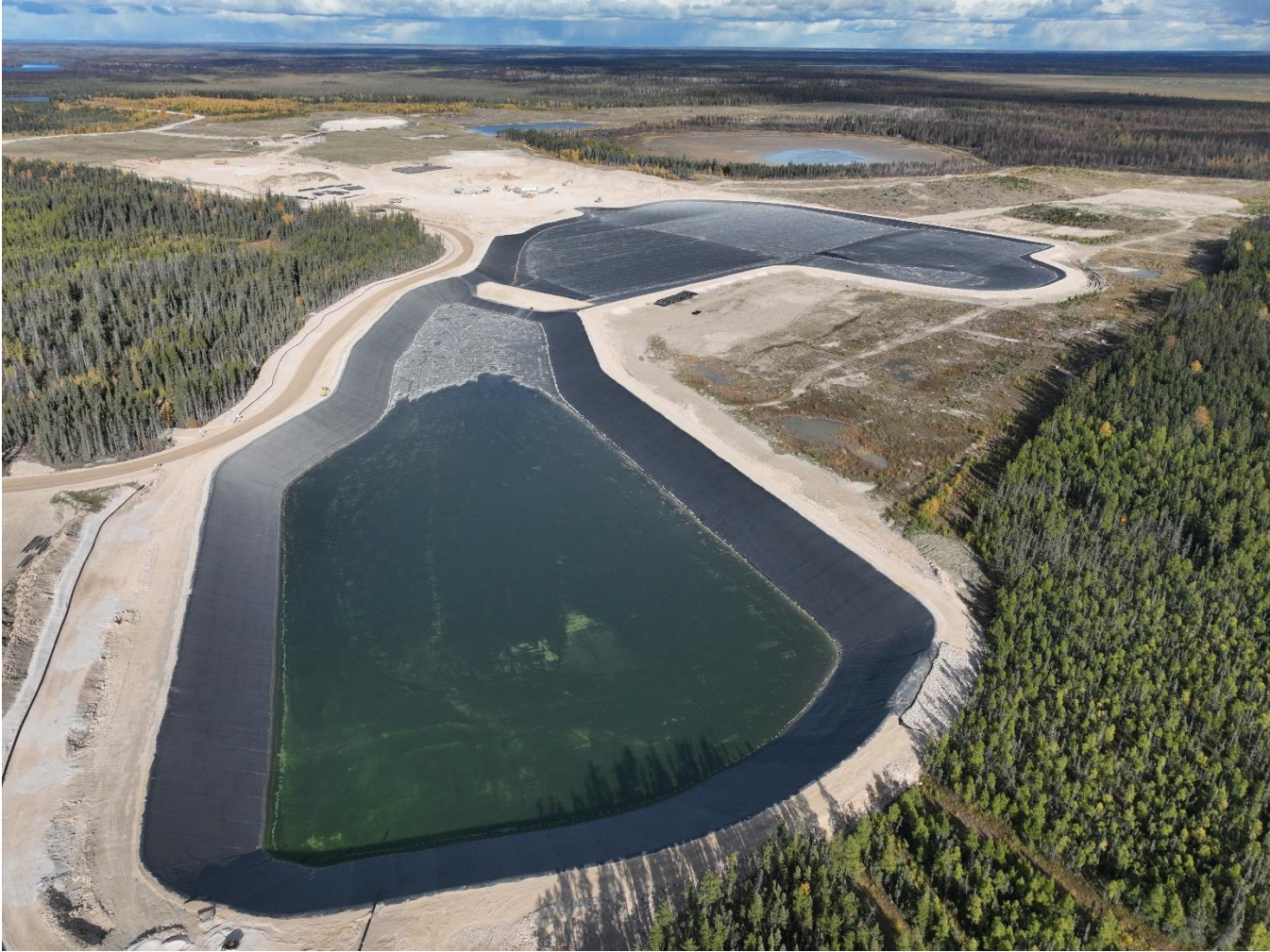
Dry Stack Tailings Area Phase 1 and Tailings Area Water Management Pond (Foreground) with Completed Liner Installation
