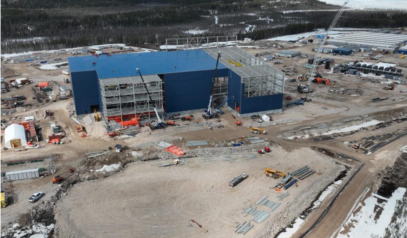
Process Plant – with Transmission Line Substation pad below
