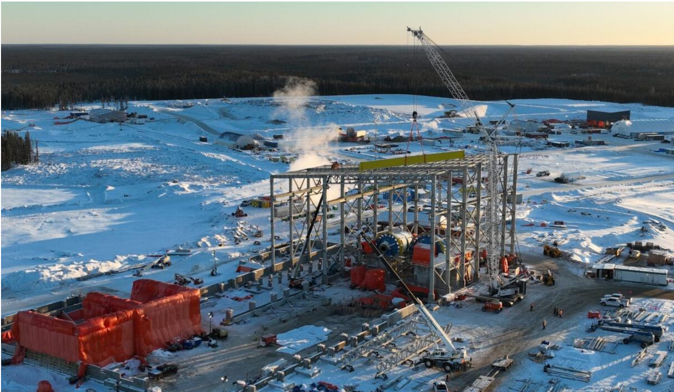
Process Plant (looking North)
